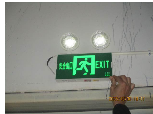
Emergency light test
