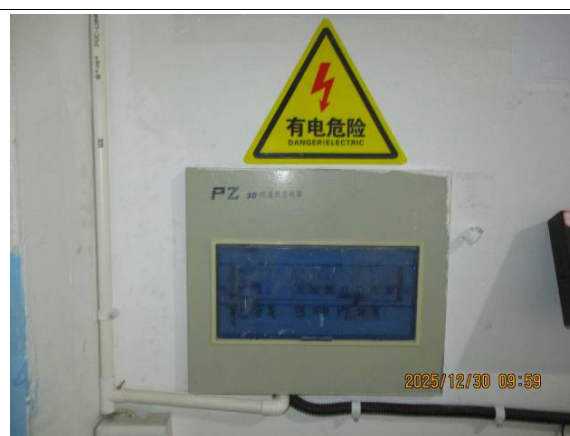
Safety electric box with warning sign
