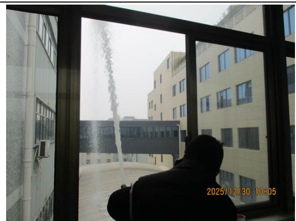
Fire hydrant test
