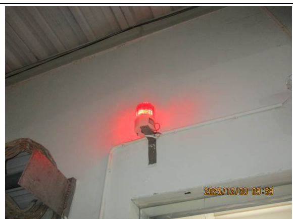
Fire alarm test
