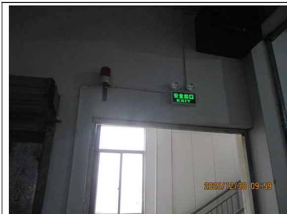
Exit sign, Emergency lamp and Fire alarm
